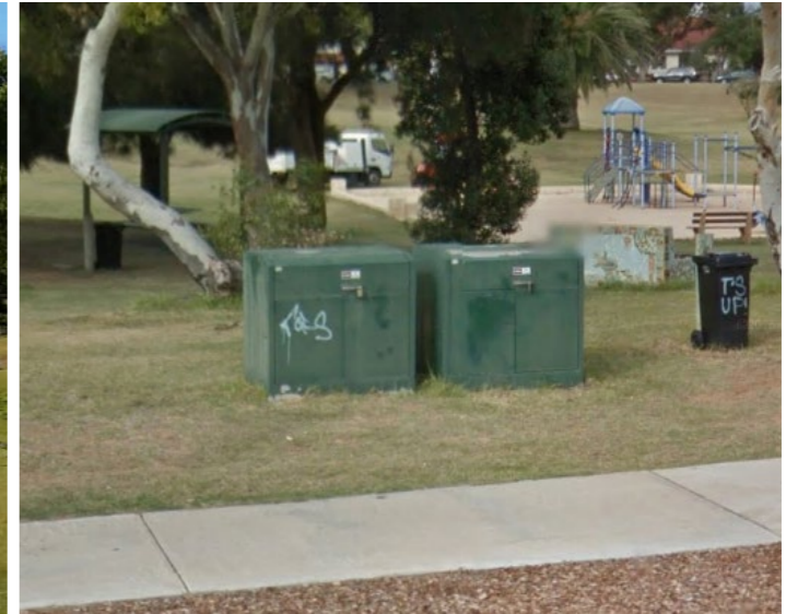
3 EXISTING ELECTRICAL SUBSTATIONS ON MAITLAND STREET
